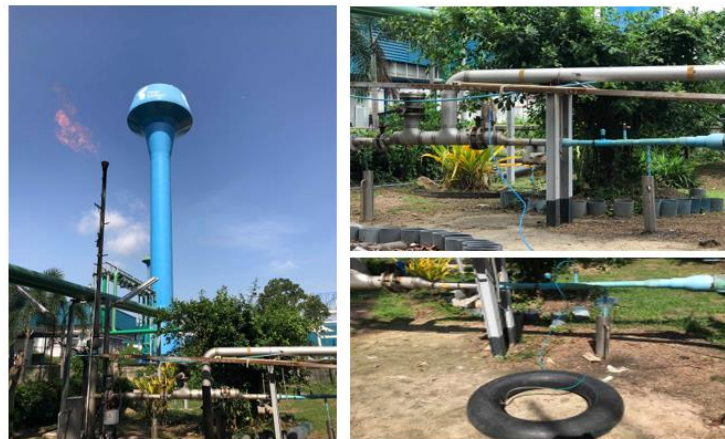
Figure 3.1 Anaerobic fermentation of wastewater treatment system.
