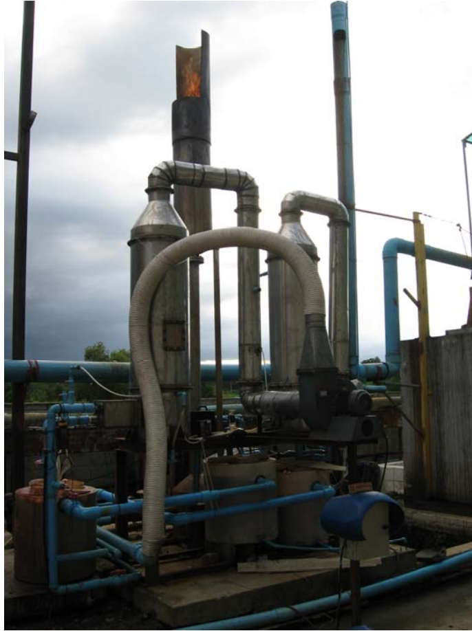
Figure 2.2 The Pilot packed column used in H 2 S removal from biogas process
