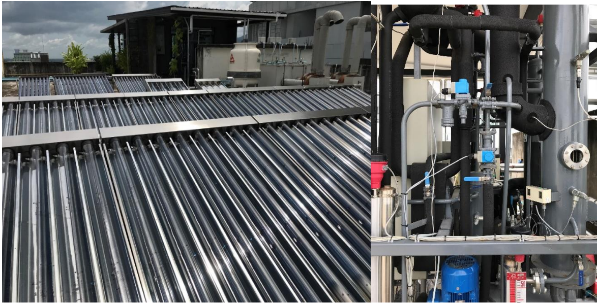
Fig. 3.3 Demonstration of Solar Cooling system at Solar Energy Research Unit, Prince of Songkla University, HatYai, Thailand.
