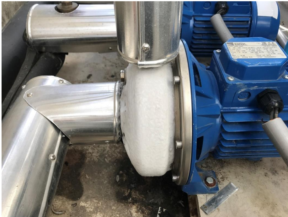
Fig. 4.18 Ice formed on chilled water pump during cooling process
