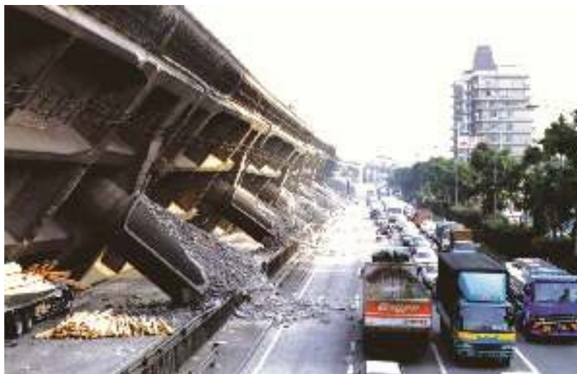
Figure 1-2 Damaged bridge piers from 1995 Kobe earthquake [Ghasemi et al., 1996]
