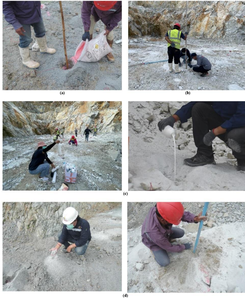
Fig. 8 Natural rubber latex blasting process (a) Charge high explosives and ANFO, (b) Load the drill cutting into the blast hole, (c) Combine natural latex with acid in a bottle, and shake before pouring into the blast hole, (d) Cover the blast hole with drill cutting.
