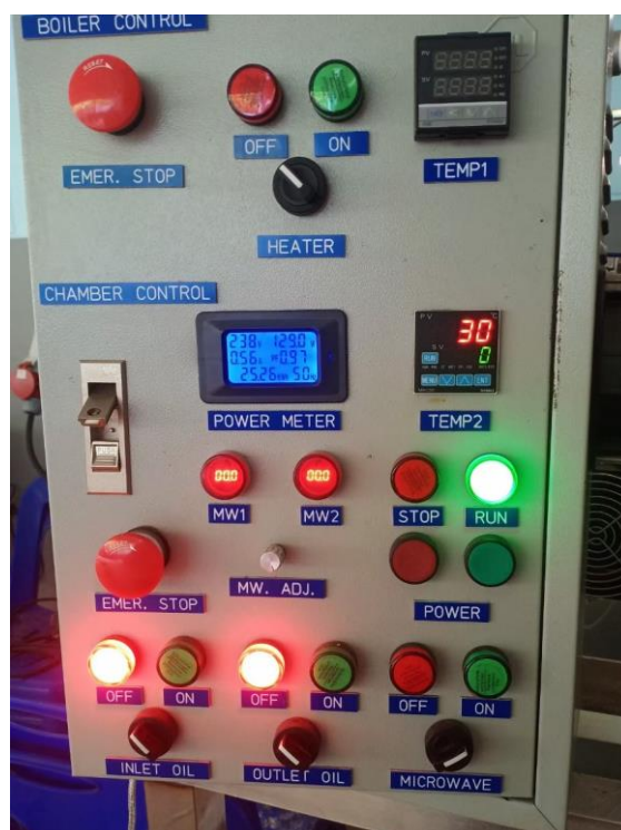
Figure A2. System electrical control box.
