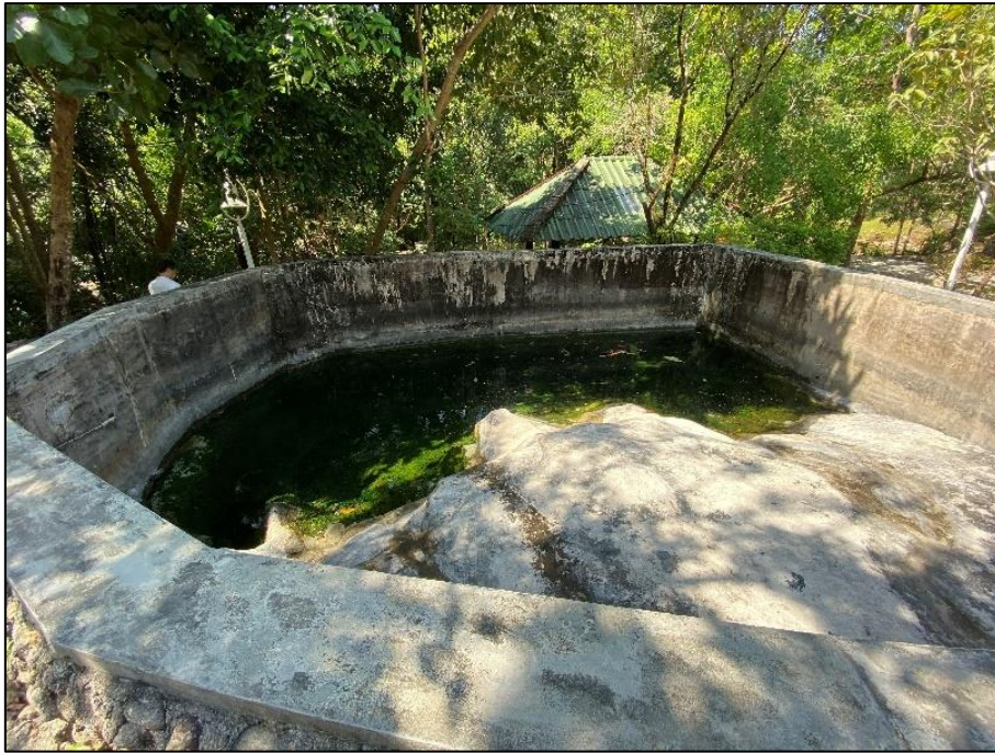
Figure 3.23 Hot spring of RN3 is surrounded by concrete structure to separate it from the waterfall.
