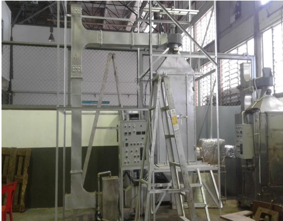
Plate A4: Fabricated rubber sheet drying system with the recirculation ducts.
