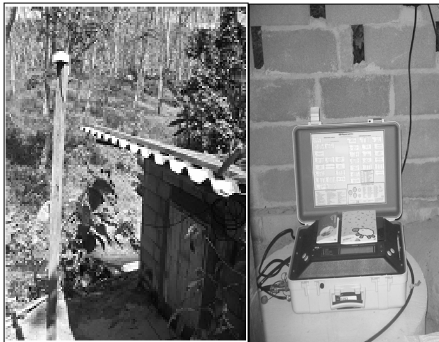
Figure 2.16 Left : Seismic station location near a small river with a small concrete shelter containing a concrete tube and the Orion portable seismograph and a GPS antenna in front. Right : Concrete shelter, where the Orion portable seismograph is protected in the concrete tube.
