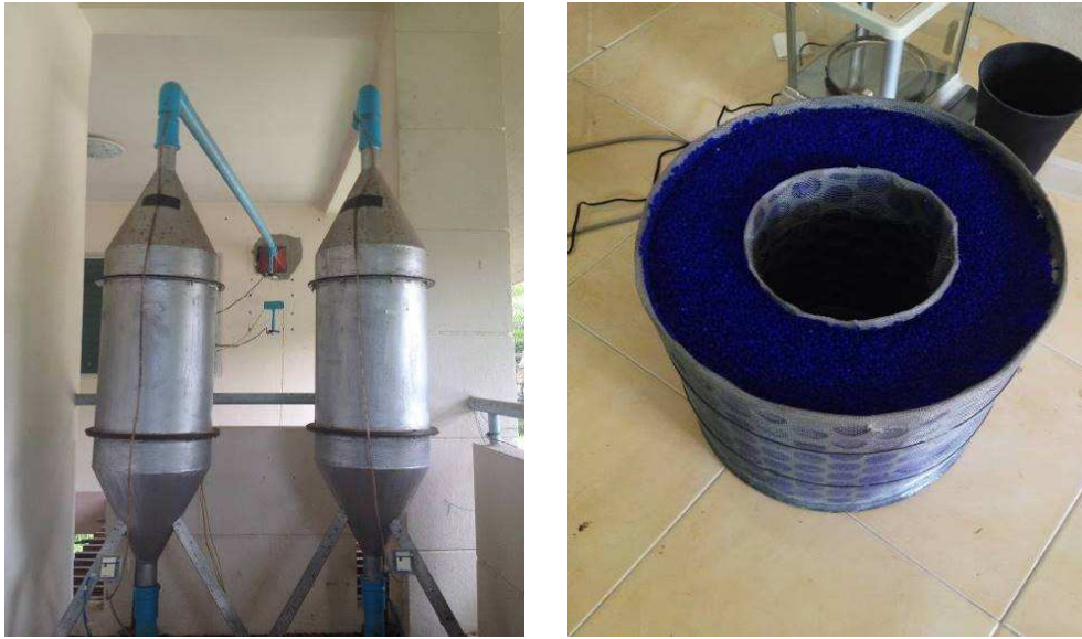
Fig. 3.5 Dehumidifiers and desiccant media
