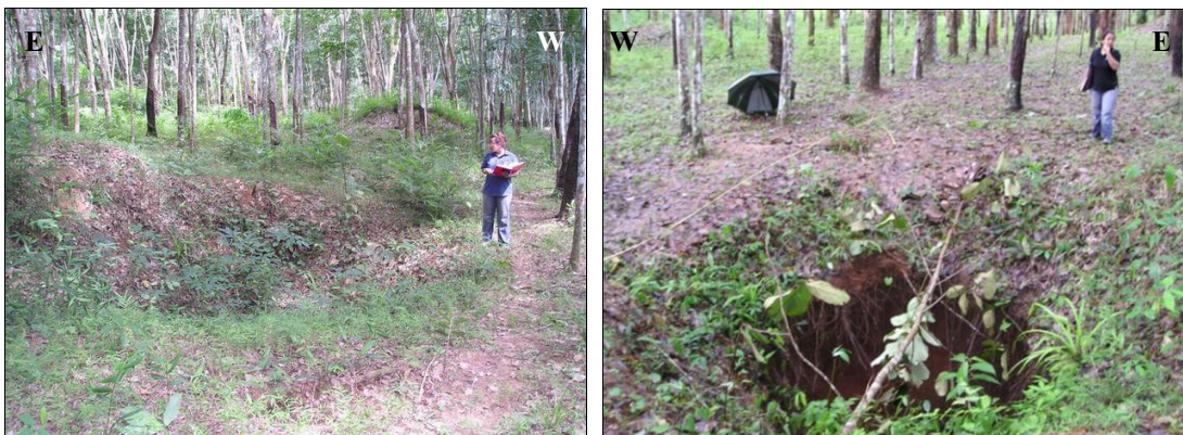
Figure 3.8 Ground subsidence observed in June 2009 (left) and the development to sinkhole in August 2009 (right).
