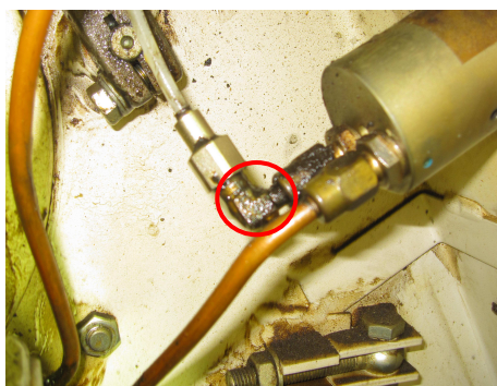
(A) Deterioration point of manual switch
