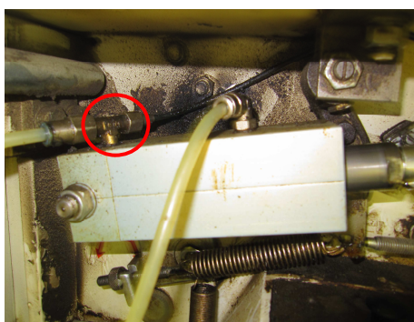
(C) Deterioration point of feed roller cylinder
