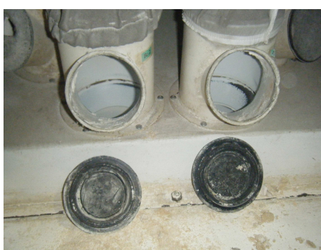
(C) Cleaning of flour transfer pipe
