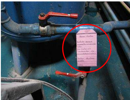
(E) Unlabeled of pipeline
