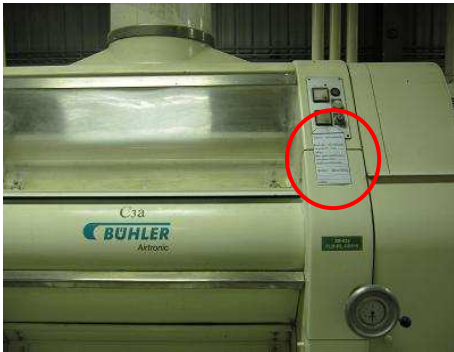
(A) Broken of ammeter dial at grinding machine
