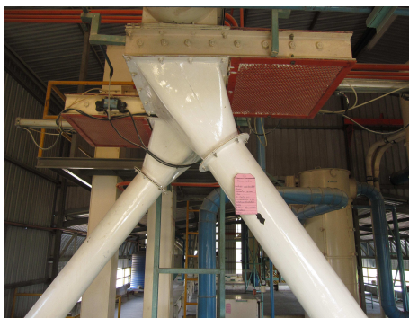
(C) Flour transfer pipe before improvement
