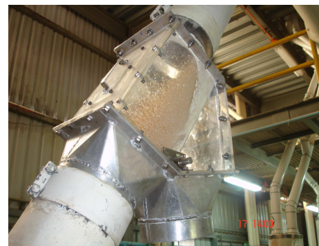
(B) Flap box of four transfer pipes after improvement
