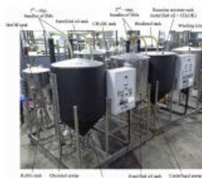
Fig. 5. Pilot-scale of two-step biodiesel production process from MCPD using the circulation process through the bundle tubes of static mixer reactor.
