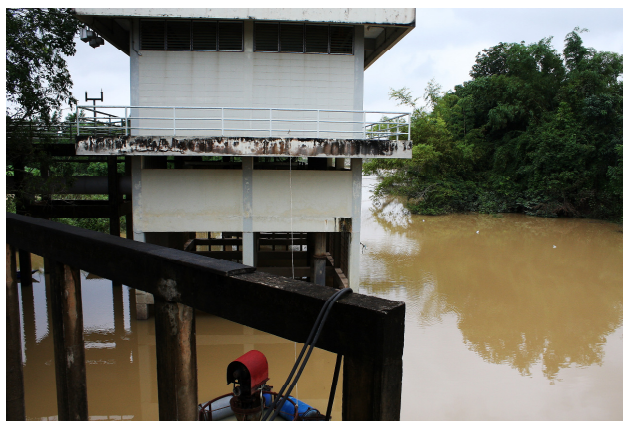
Figure 3.1 Pumping Station of Hat Yai, Songkhla, province, Thailand
