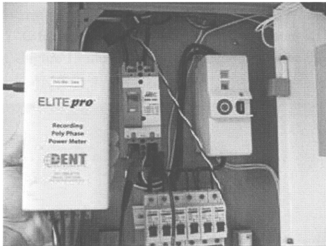
Figure 11 Continuous power meter
