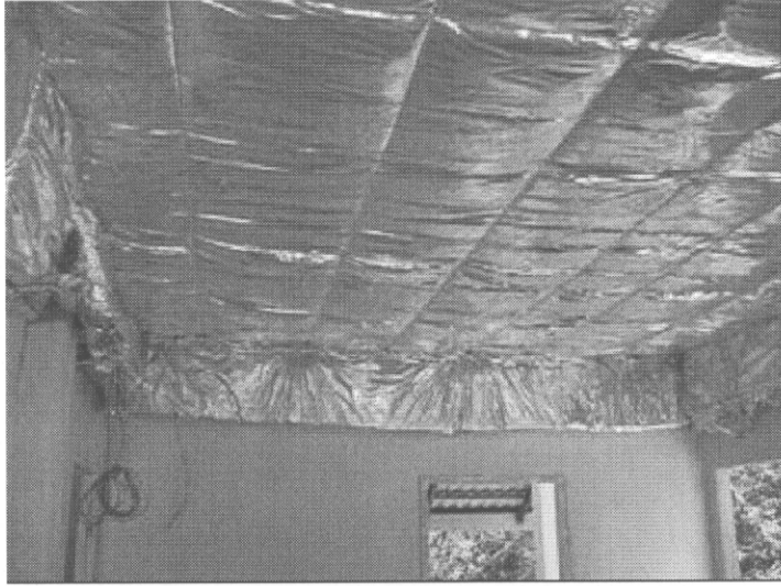
Figure 18 Fiber glass insulation
