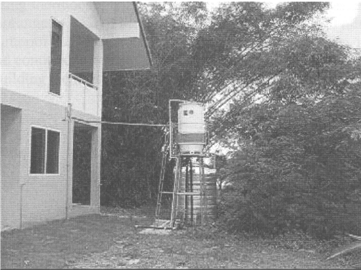
Figure 21 Cooling tower, storage tank and piping system
