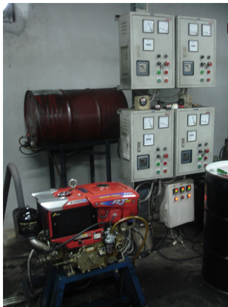
Figure 3.4 The engine and the generator used in this work.
