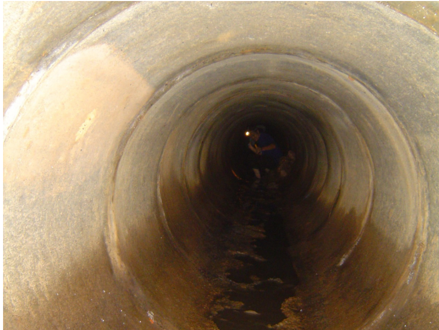
Figure 6. The concrete conduit near headquarter of Chiang Dao Wildlife Sanctuary, Chiang Mai which the bats live in.
