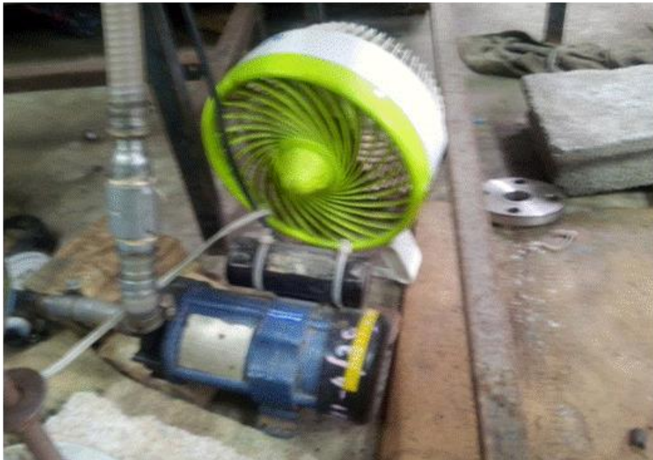
Figure 66 Centrifugal circulation pump and cooling fan.
