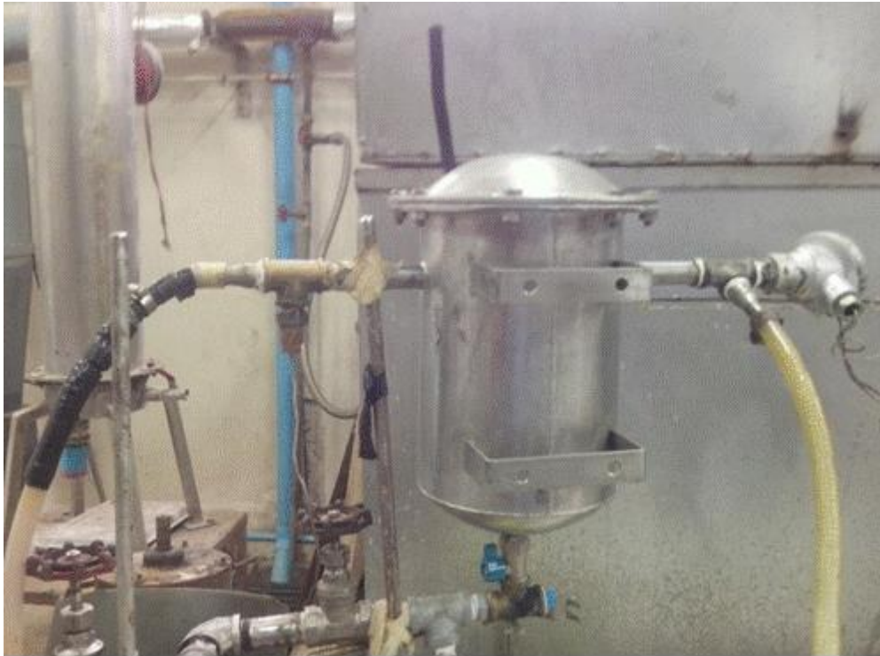
Figure 64 Liquid-gas separator with temperature sensor.
