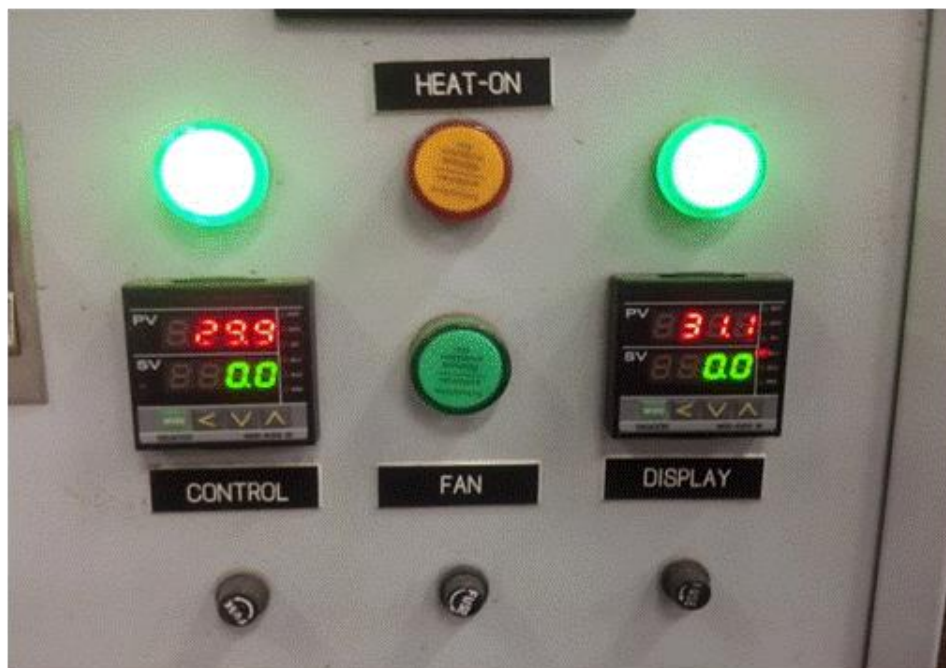
Figure 67 Temperature control panel.
