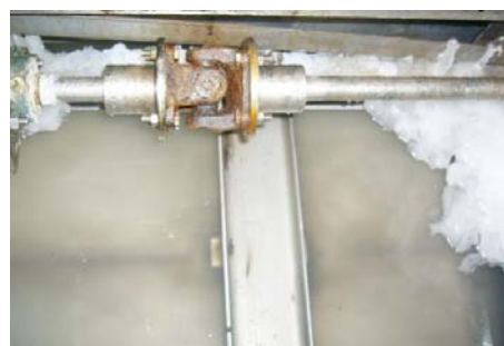
The ice inside brine tank
