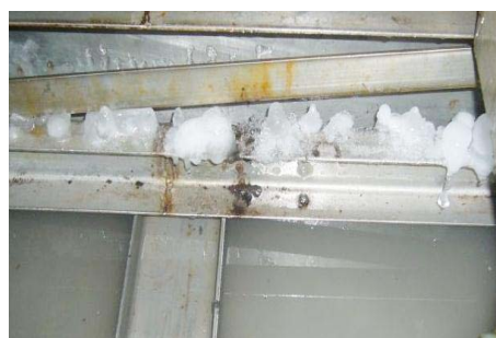
The ice inside brine tank
