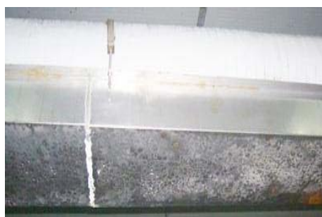
Dropping of water on the gutter
